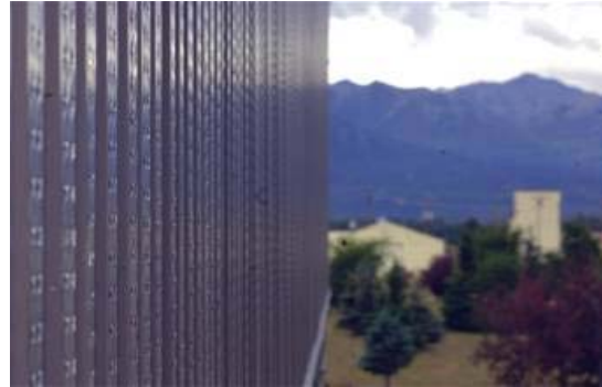
ELMENDORF AIR FORCE BASE, Alaska -- In November 2008, Elmendorf was the location for Alaska and Pacific Air Forces to install solar walls. Two of these walls hang on the outside of the 3rd Logistics Readiness Squadron, so far they have saved Elmendorf $15,000 in energy cost. (U.S. Air Force photo/Airman 1st Class Christopher Gross)
