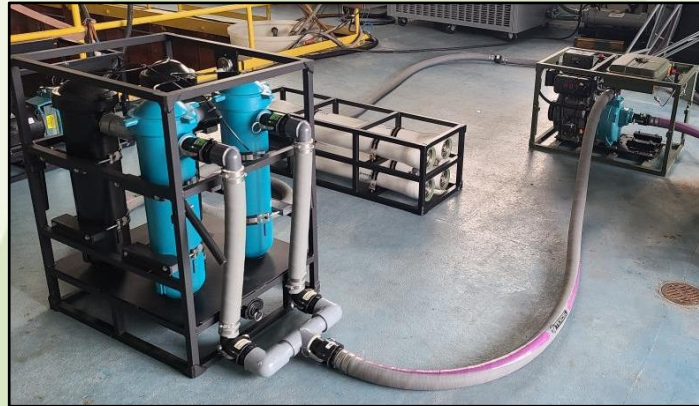
Graywater Recycling Pretreatment System
