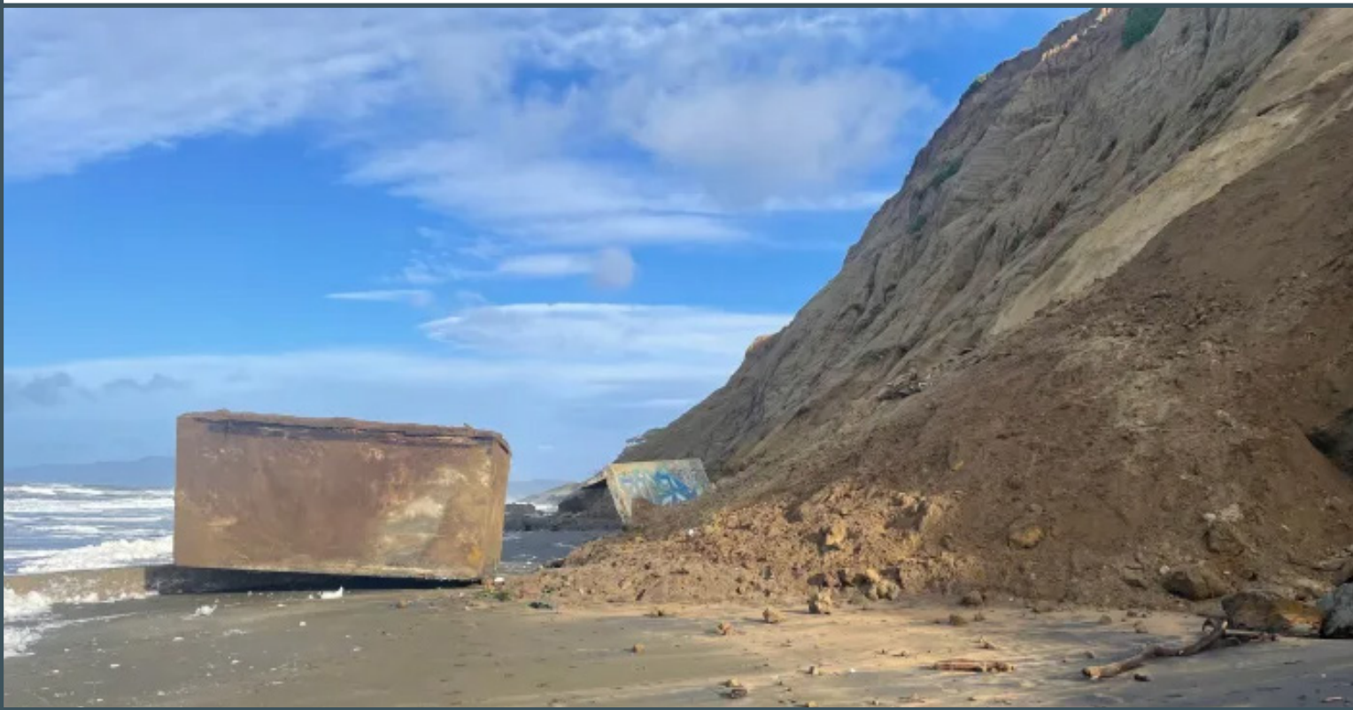
A World War II bunker tumbled down a cliff on California beach, 2022 (Source: Yahoo News, Photo credit: National Park Service, Golden Gate National Recreation Area)
