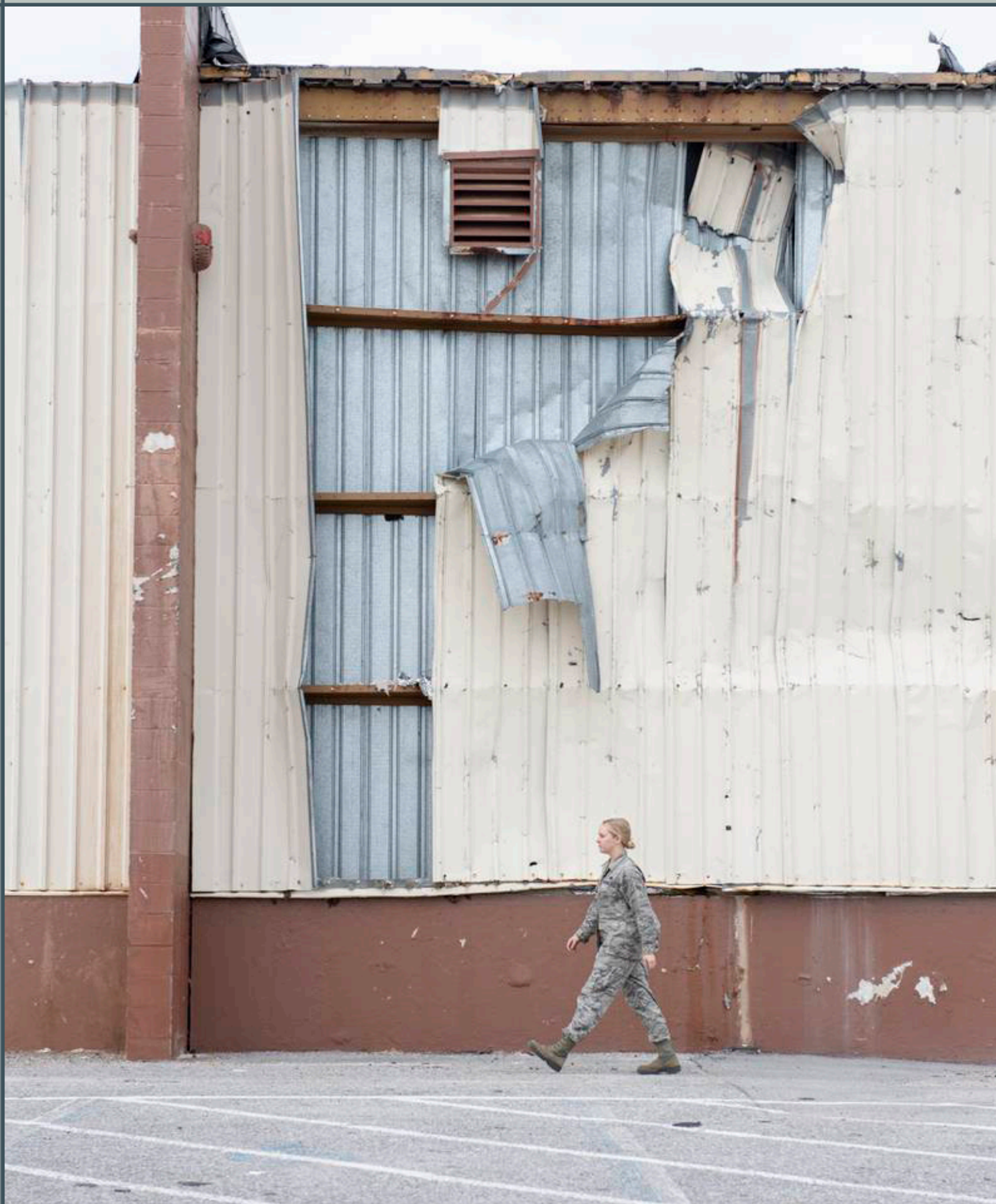
An Airman walks past the 325th Logistics Readiness Squadron materiel management flight warehouse at Tyndall Air Force Base, Florida, which was damaged by Hurricane Michael, March 13, 2019 (Source: Senior Airman Javier Alvarez/U.S. Air Force)
