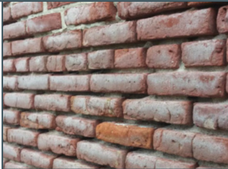
Effects of Hurricane Sandy on masonry in Crisfield, Maryland, 2012 (Source: Lisa Craig)
