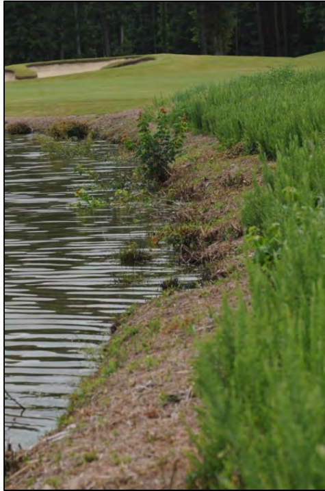
Vegetation control border at pond 0 and associated erosion.
