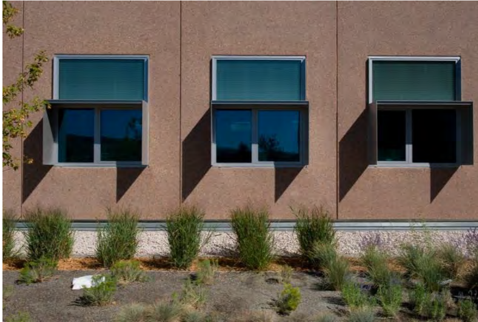
Shading was applied around the windows on the exterior of the Research Support Facility (RSF) at the National Renewable Energy Laboratory (NREL) to reduce glare and overheating of the building interior. These windows are also bird friendly. Photo by Dennis Schroeder, NREL 19798
