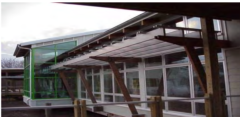
Window netting installed feet from window on slanted wooden beams. Photo by USFWS
