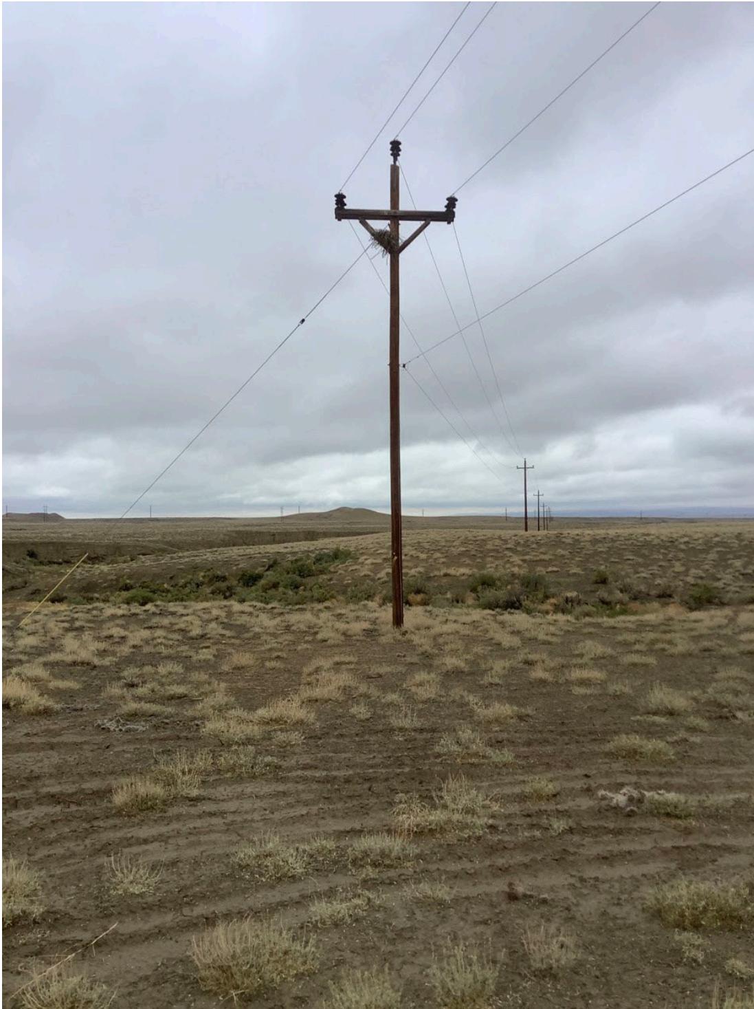
Figure B-11. Power Pole Nest at the Lovell LTA
