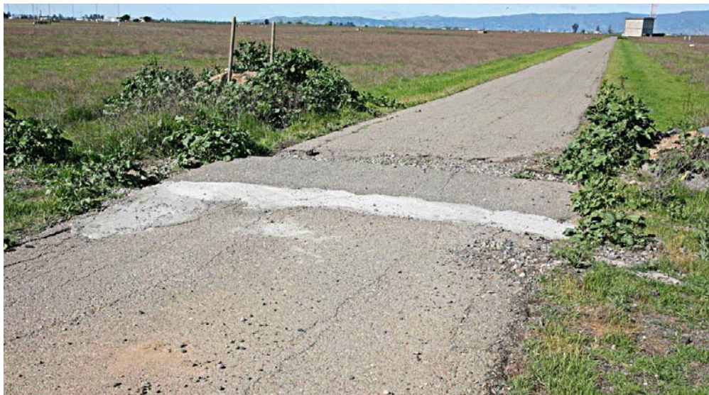
Figure 18. Ground squirrel damage to an antenna access road. Note concrete patch between constructed mounds with artificial burrowing owl burrows.
