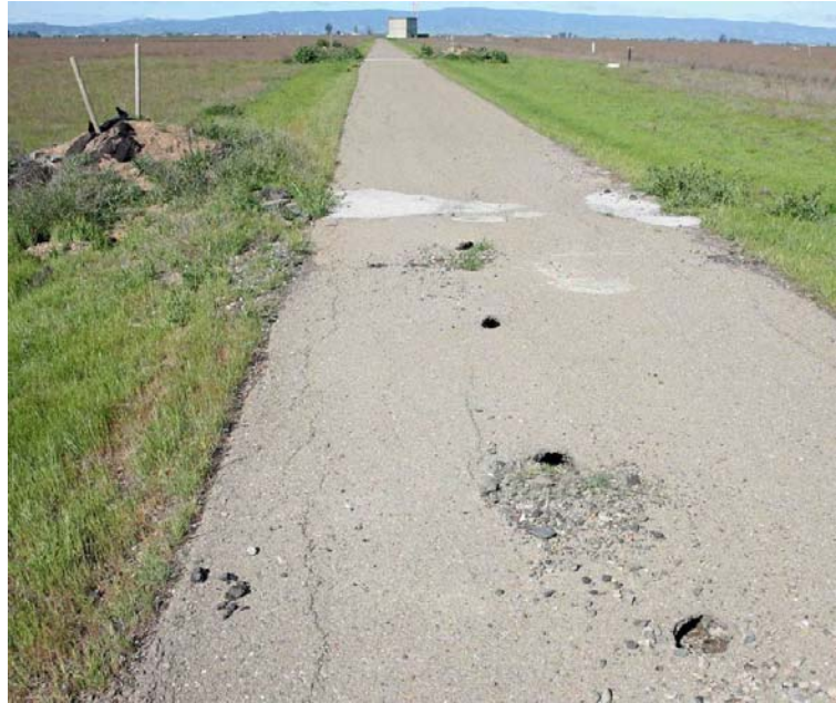
Figure 17. Ground squirrel damage to an antenna access road. Note burrow entrances in middle of road, and concrete patches between constructed mounds with artificial burrowing owl burrows in background.
