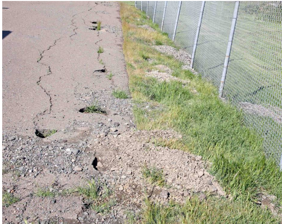
Figure 19. Ground squirrel damage along the edge of an asphalt pad of the main transmitter facility. Note cyclone fence falling over, and note constructed mound with artificial burrowing owl burrows in background (top right corner of photo).
