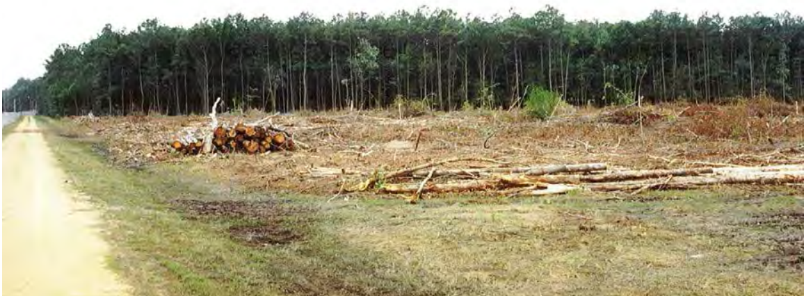
Runway clearing project at Webster Field Annex: An illustration of the Management Practices and Prescriptions (MPPs).
