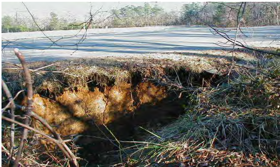
Example of erosion at NAS PAX: Stormwater management will help remedy similar future impacts.
