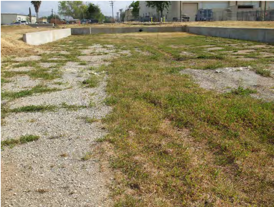
Photo 6 (April 2009): Open concrete basin (Pond #17) at the beginning of the main drainage channel through Survey Area 13. Sediment collected over the gravel base and wetland plants (dominated by Bermuda grass) are growing in the sediment. This is man-made feature and did not meet the criteria for determination of wetlands
