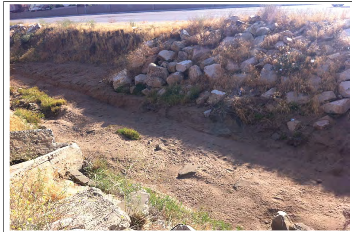
Photograph 4: View looking northeast, just north of Meyer Drive. The photo represents area of unvegetated streambed within Heacock Channel upstream of Meyer Drive.
