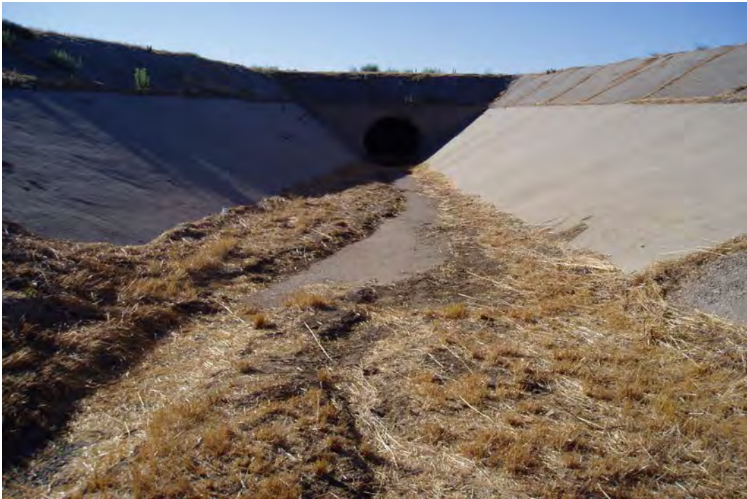
Photo 5 (October 2006): Concrete lined channel in the main drainage in Survey Area 13. Debris and sediment collected at the base of the channel and patches of wetland plants had established on top of the sediment. Water flows into an underground culvert at the end of this channel (slightly visible in the shadow).
