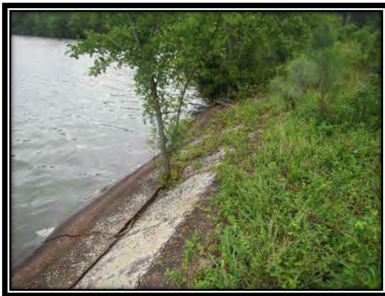
Vegetation Encroachment on Lower Big Bethel Dam
