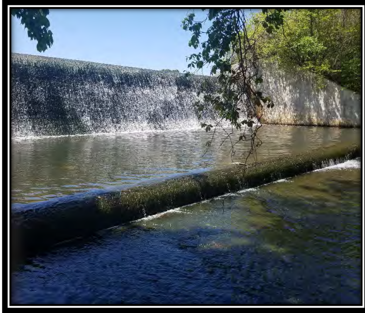
Lower Big Bethel Dam in Need of Repair
