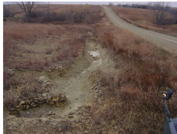
Figure 6: Maneuver damage in a drainage ditch that is eroding away to become a gully
