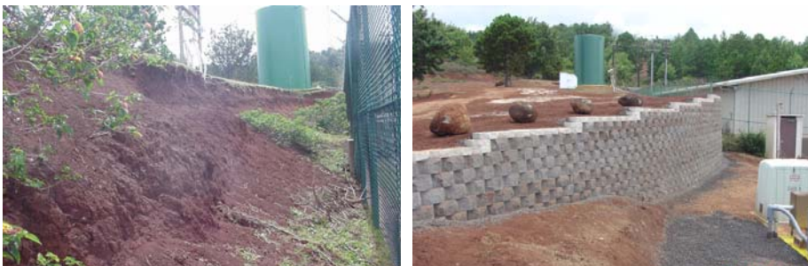
Photo 4-10: A developed portion of Mākaha Ridge Tracking Station before and after the construction of a retaining wall to protect site structures.
