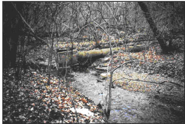
Photo B - Large section of storm sewer undercut and exposed by erosion and slope failure.
