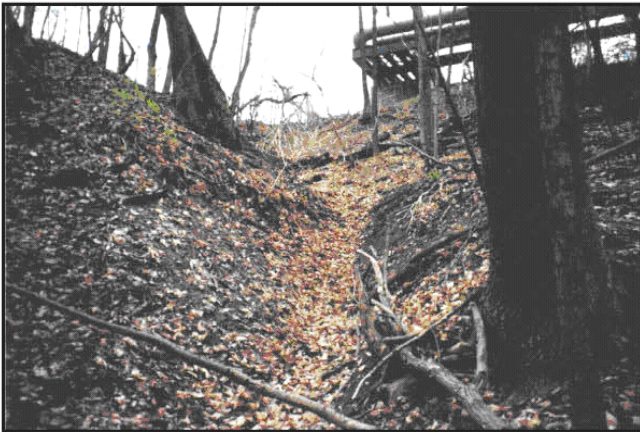
Photo A - Erosion in Pettibone Ravine resulting from storm water runoff being direct into the ravine instead of a storm sewer.
