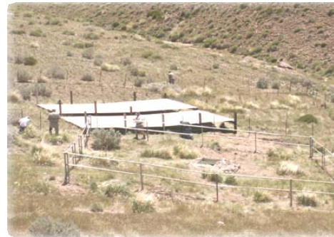
Guzzler installed on the east side of Fairview Peak in 2010. Fence was erected to keep livestock out.
