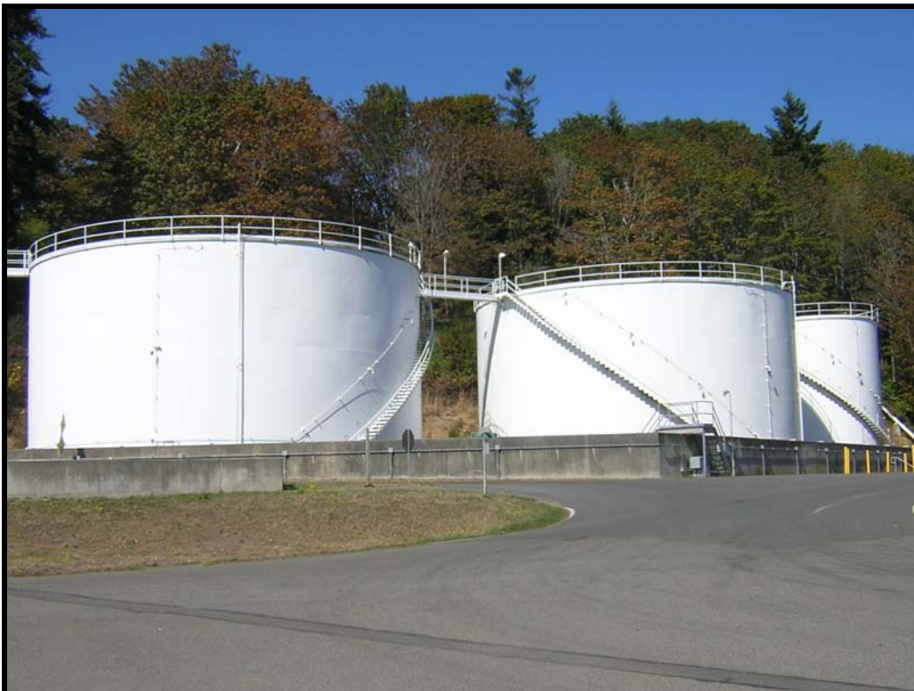
Figure 2-2. Manchester Fuel Department – Oily Wastewater Tanks.
