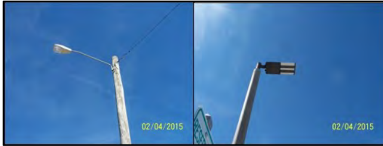
Figure 6. Arm-mounted area “cobrahead” light fixtures observed at Joint Expeditionary Base Fort Story
