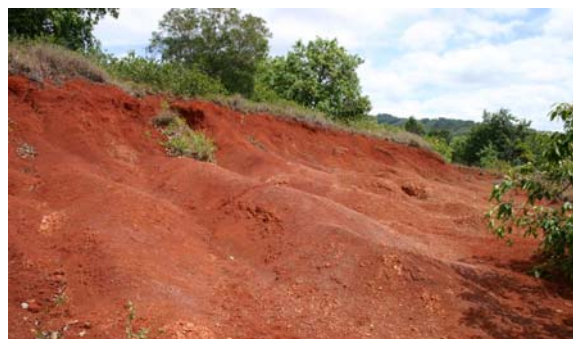
Photo 3-8: Soil erosion at Red Hill Fuel Storage Area
