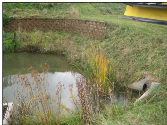
Area 4 – Stormwater Detention Pond
