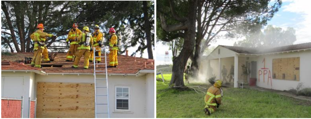
Photo 8. Structural firefighter training prior to demolition of old housing buildings, 2011. (Photos by C.M. Wolf)
