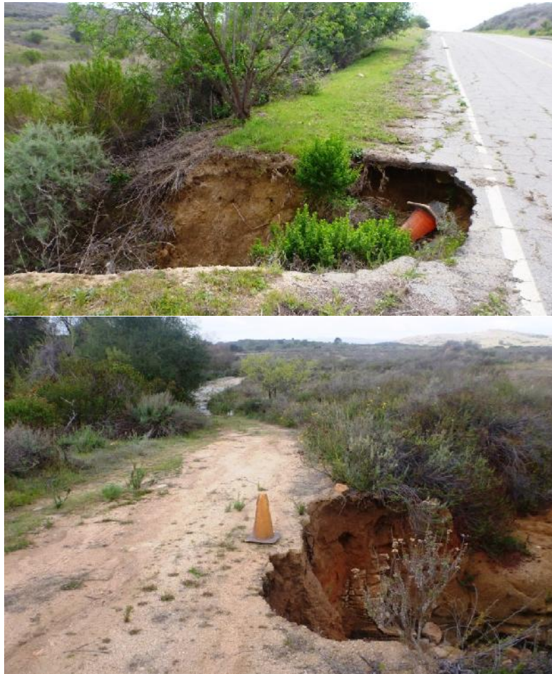
Photo 43. Soil erosion not only threatens infrastructure such as the roads shown here, but also natural resources. (Photos by AMEC 2013).
