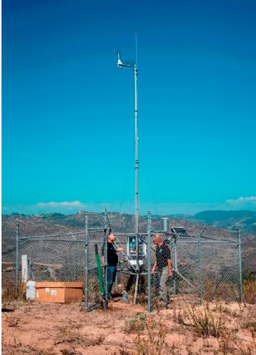
Photo 39. Installation of RAWS weather monitoring tower. (Photo by MCI Eli J. Medellin)
