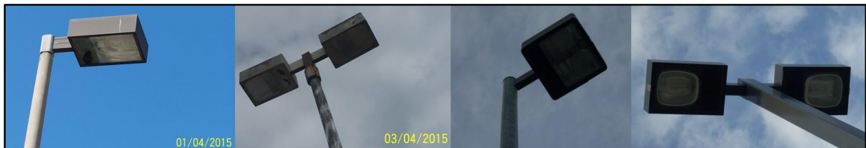
Figure 5. Typical arm-mounted cutoff - shoebox fixtures identified at Naval Air Station Oceana – Dam Neck Annex.
