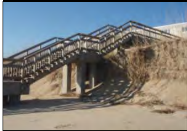
Eroding sand dunes at Dam Neck Annex (February, 2010)
