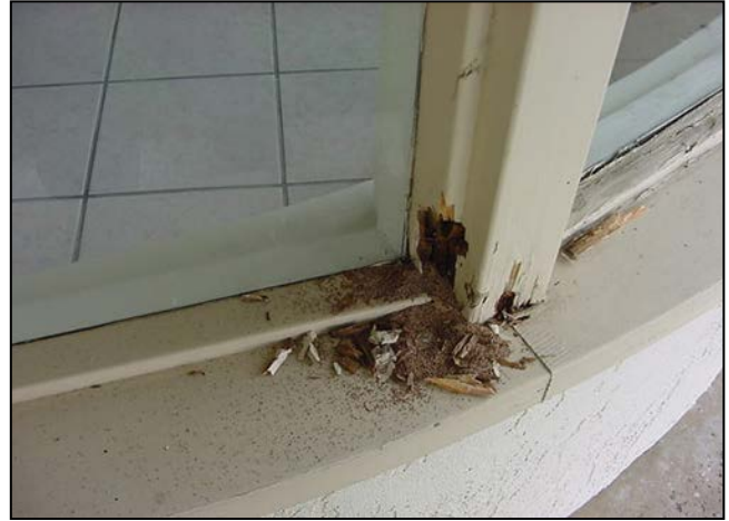
Drywood termite damage.
