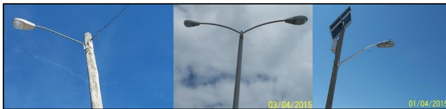
Figure 4. Typical arm-mounted area – cobrahead fixtures identified at Naval Air Station Oceana – Dam Neck Annex.
