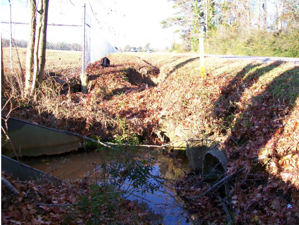
Photograph 5-23: NASO 20, Ditch Scour and Embankment Erosion at Outfall 005
