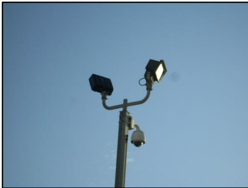
Figure 12. Perimeter flood lighting used at Naval Air Station Oceana – Dam Neck Annex, Naval Special Warfare Development Group Compound
