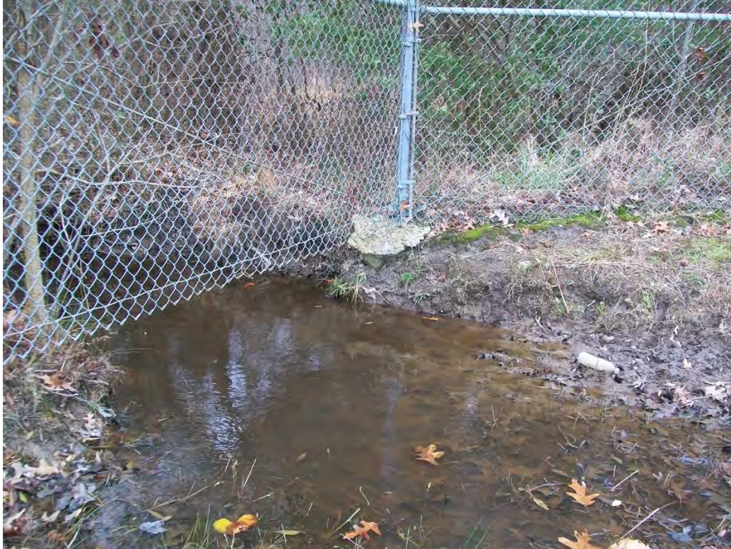
Photograph 5-24: NASO DNA 01, Streambank Scour along Roadside Ditch
