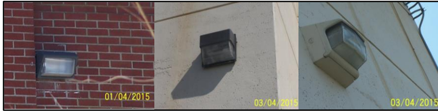
Figure 6. Typical wall-mounted area “wall pak” fixtures identified at Naval Air Station Oceana – Dam Neck Annex.
