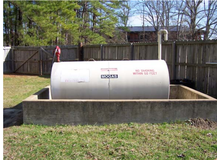
Proper signage and spill containment characterize the above ground fuel storage tank.
