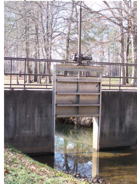
Spill gate installed near hole 4 prohibits spills from leaving the installation in emergencies.
