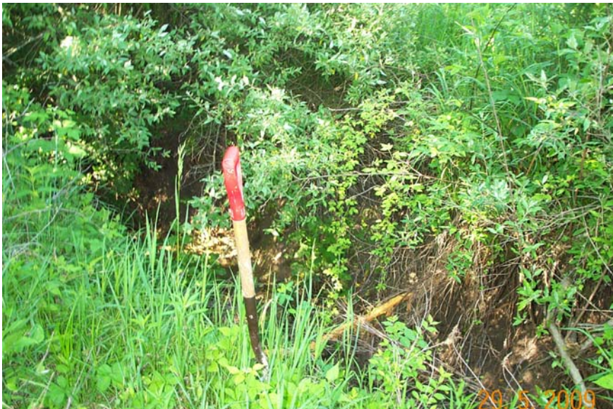
Exposed drainage tile & associated head-cut outlet.
