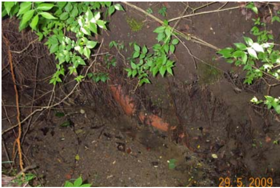
Photo 5 Gully w/ exposed tile (east side)
