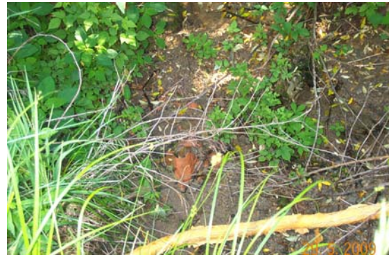
Photo 6 Gully w/ exposed tile (west side)
