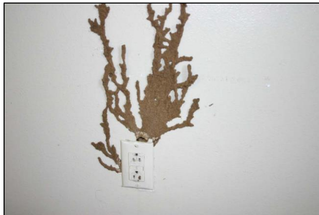
Subterranean termite shelter tubes.
