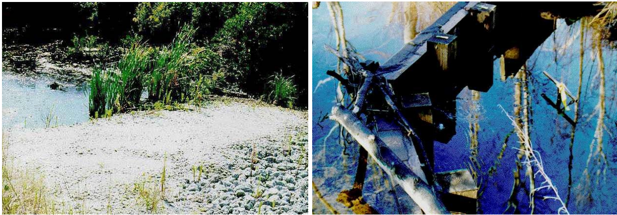
Figure 4-41. (Left) Ditch Plug in the Pocosin Area. Figure 4-42. (Right) Timber check dam in Big Shakey Swamp
