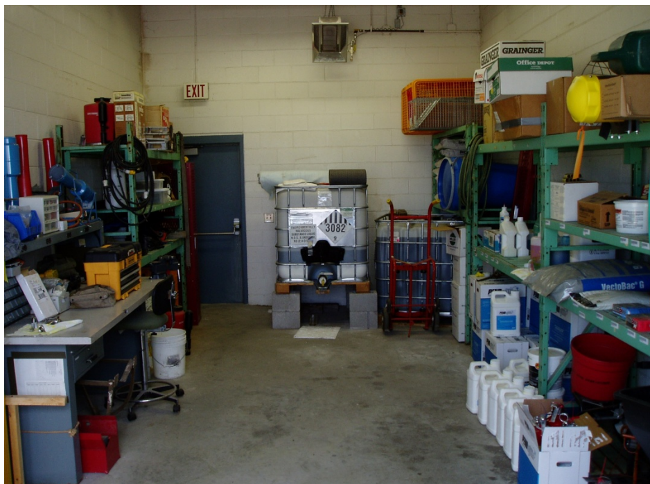
FIGURE 6.2. PEST MANAGEMENT SHOP CHEMICAL STORAGE ROOM
