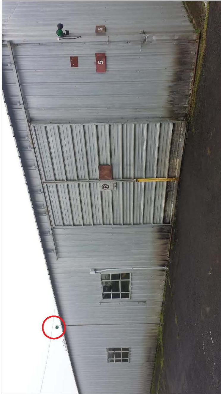
Building 5_Flood Light 4: One green bulb with no shielding and no motion detection, bulb is facing northeast and mounted onto of the top of the building.
