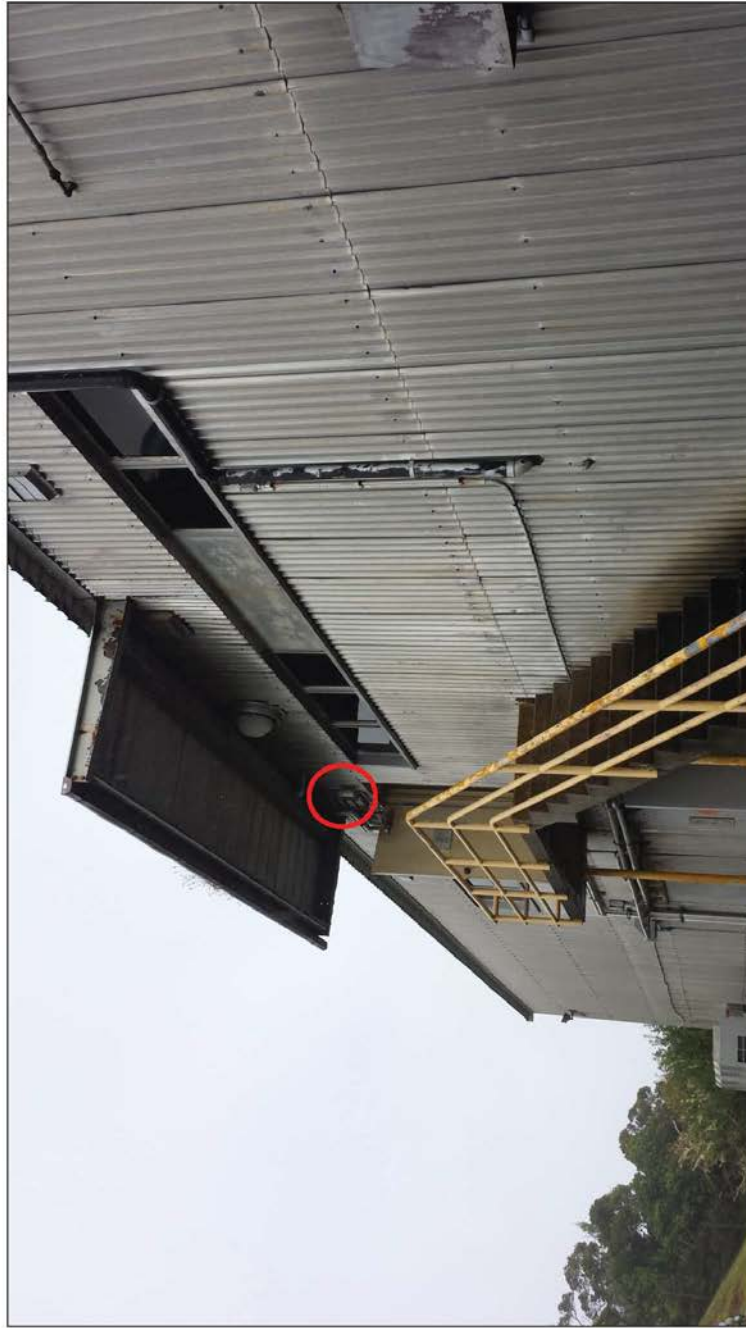
Building 1_Entryway Light 1: One white bulb, no shielding and no motion detection, 2 nd floor.
