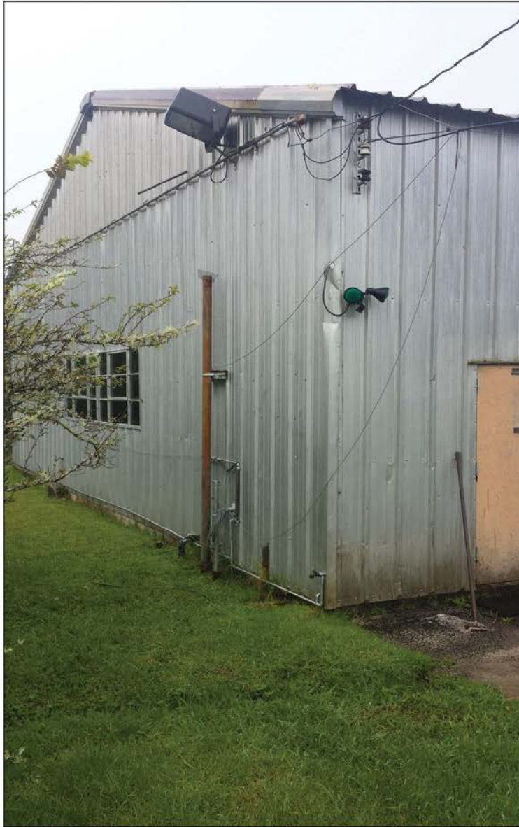
Perimeter Light_P: One green bulb, with full shielding, light is mounted to the southeast corner of building 5.
