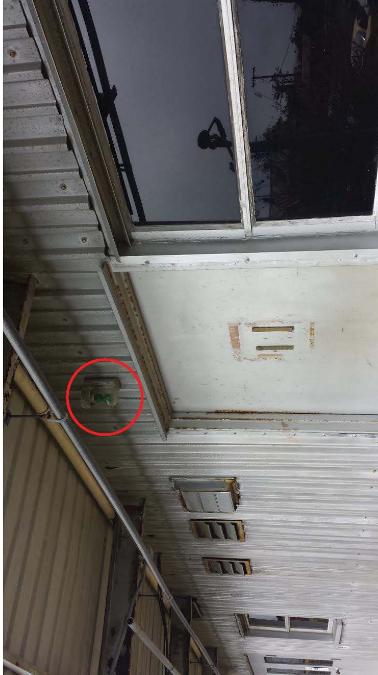
Building 1_Entryway Light 3: One green bulb with no shielding or motion detection, 1 st floor, southeast facing.
