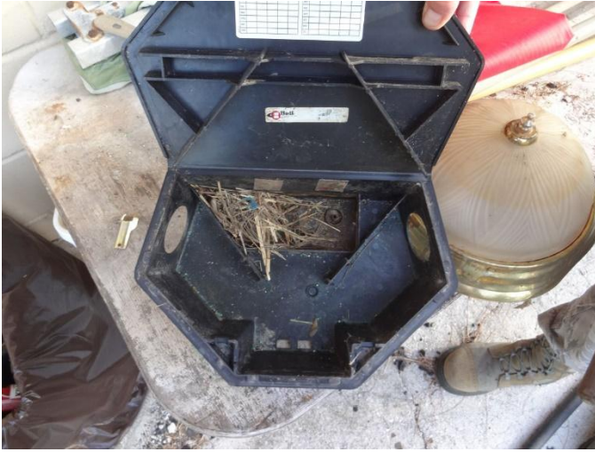
An example of a rat nest inside a bait station. Location: Arrestor cable shack.
