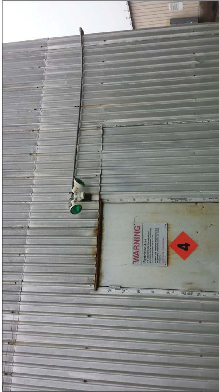
Building 1_Flood Light 2: Two green bulbs with motion detection (close-up).
