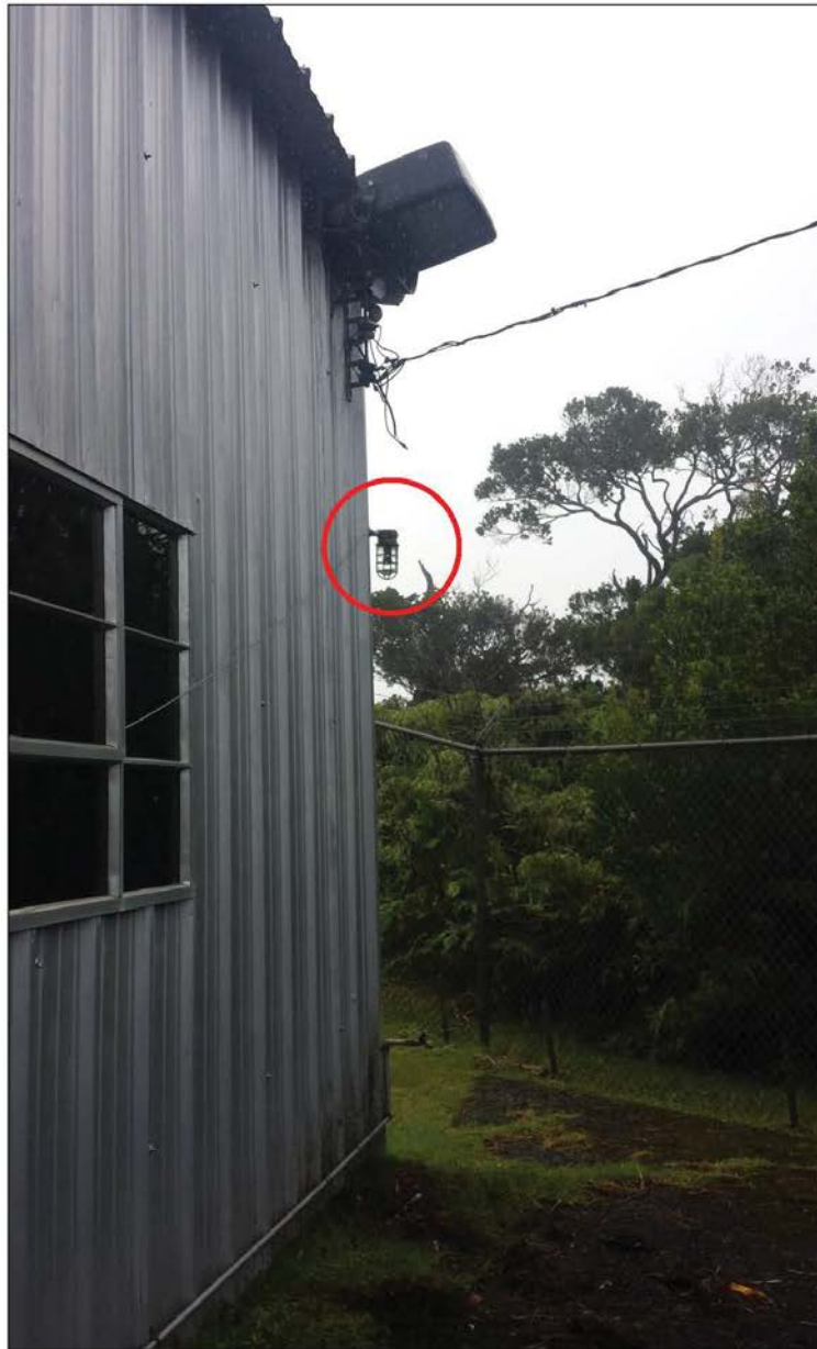
Building 5_Building Exterior Light 1: One green bulb with no shielding and no motion detection .
