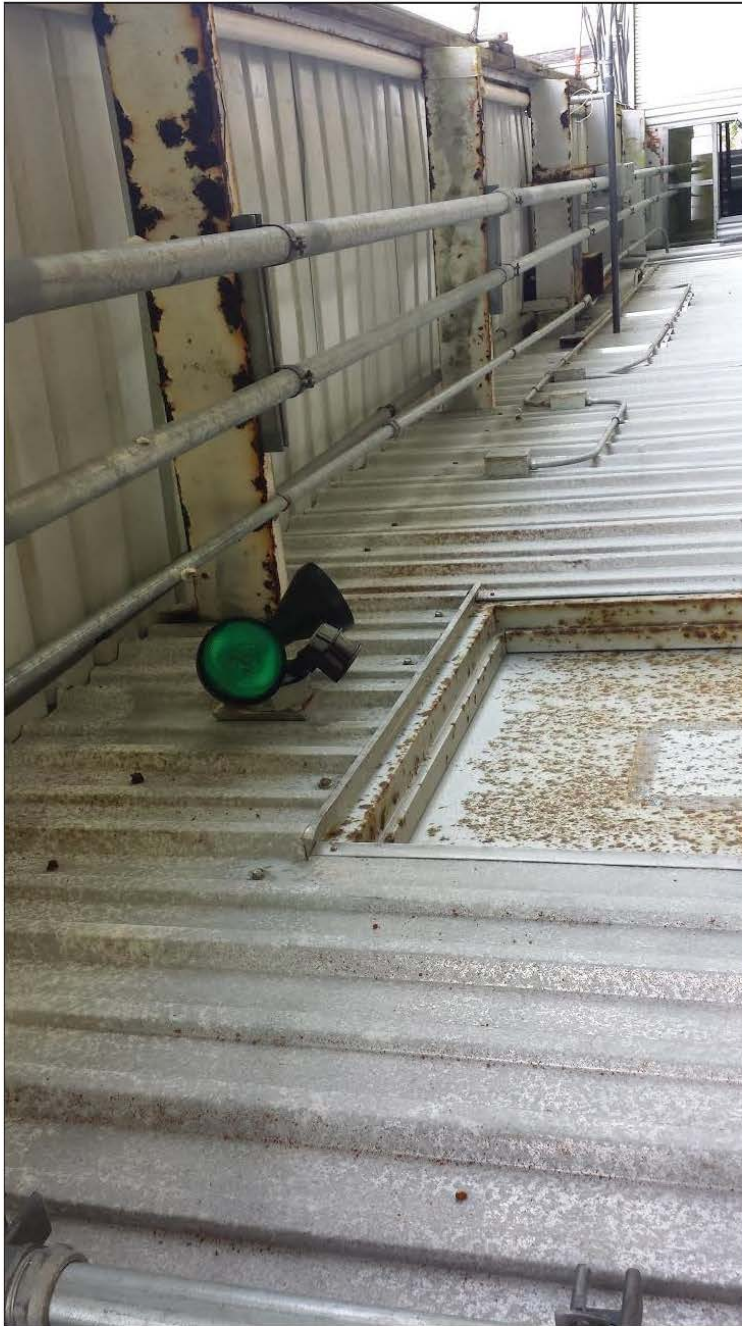
Building 1_Flood Light 3: Two green bulbs with motion detection (close-up)
