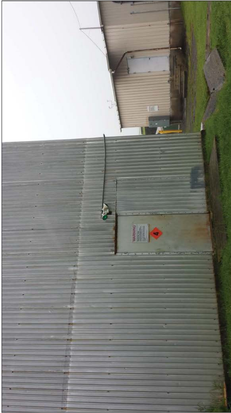
Building 1_Flood Light 2: Two green bulbs with motion detection located on the northside of the building.
