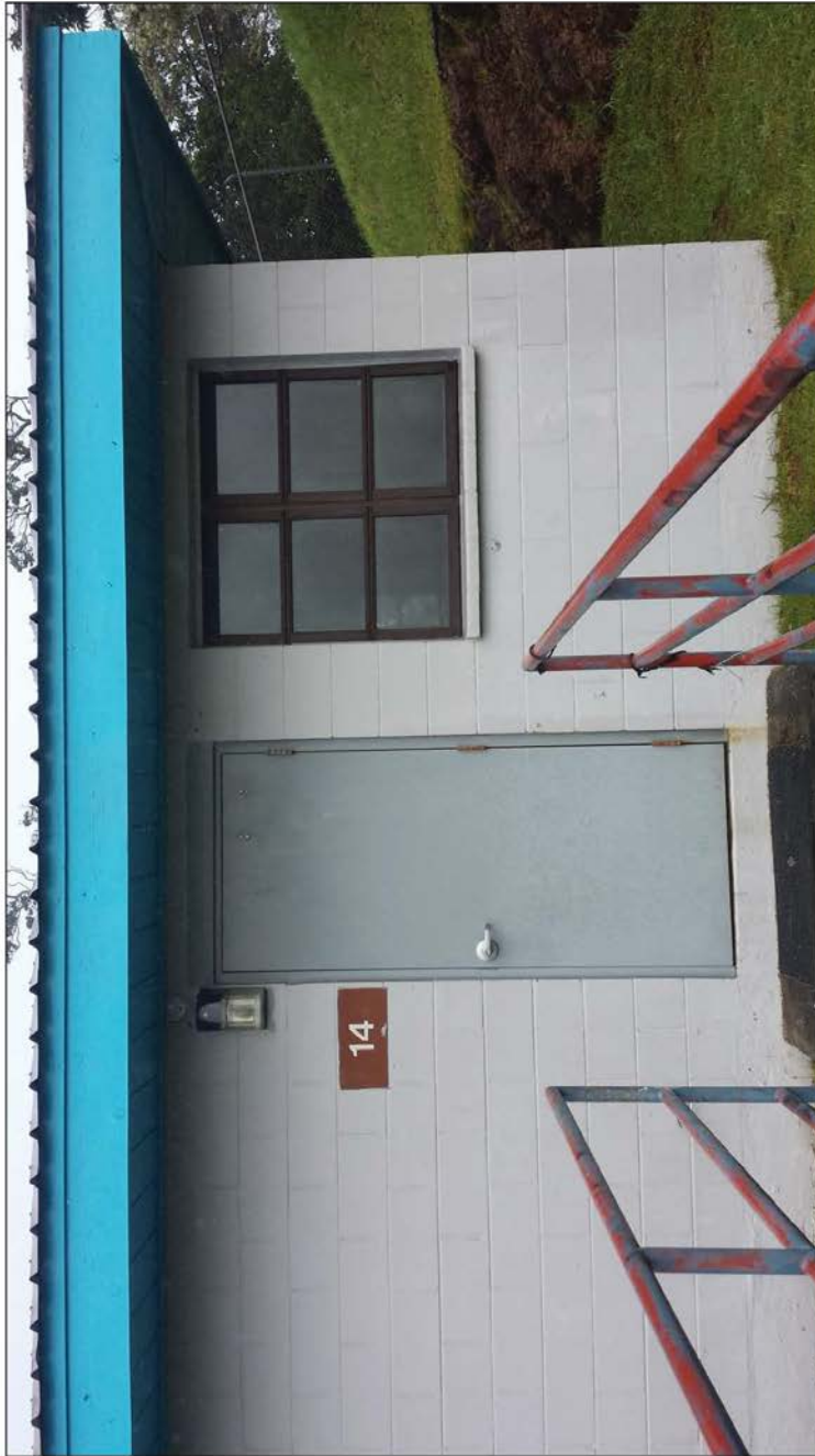
Building 14_Entryway Light 1: One white bulb with no shielding and no motion detection, southeast facing.
