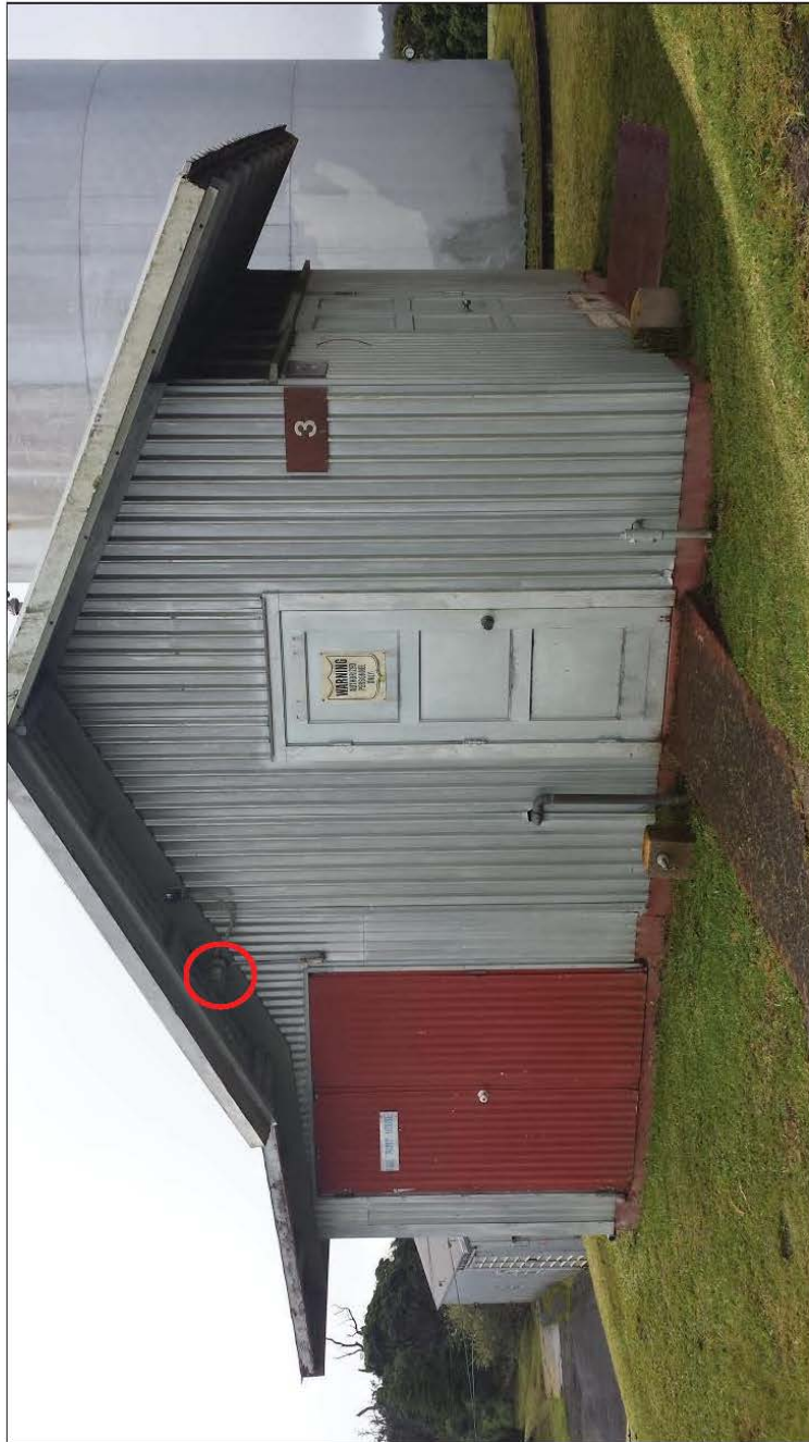
Building 3_Building Exterior Light 1: One white bulb with no shielding and no motion detection, facing northwest.
