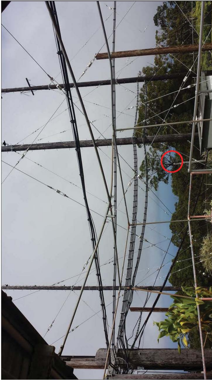
Perimeter Light_E (broad view): One green bulb, with full shielding.
