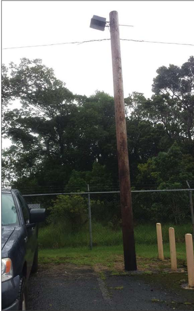
Perimeter Light_B1: One green bulb, with full shielding (light is currently not functioning).
