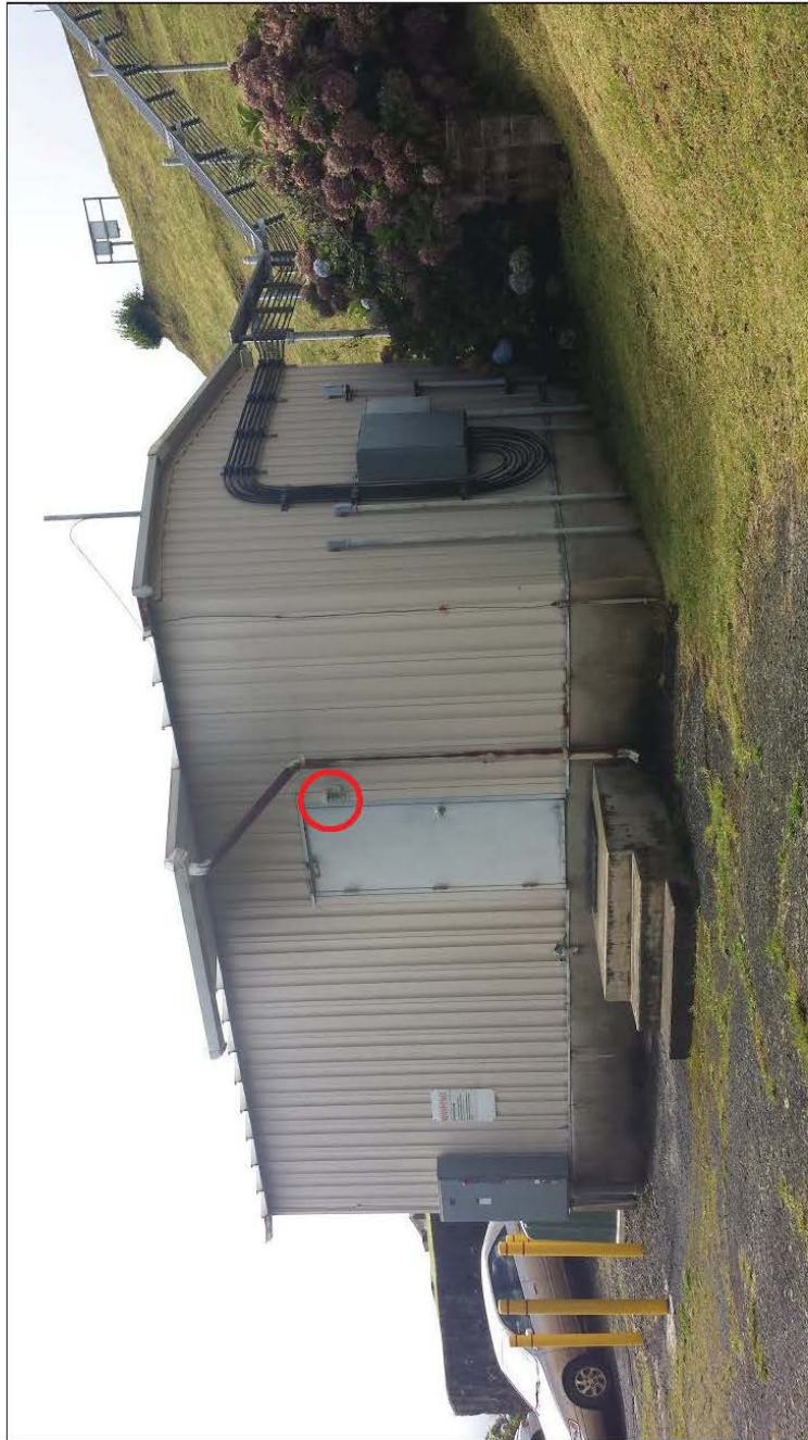
Power Shed (no building number)_Entryway Light 1: One green bulb with no shielding and no motion detection.
