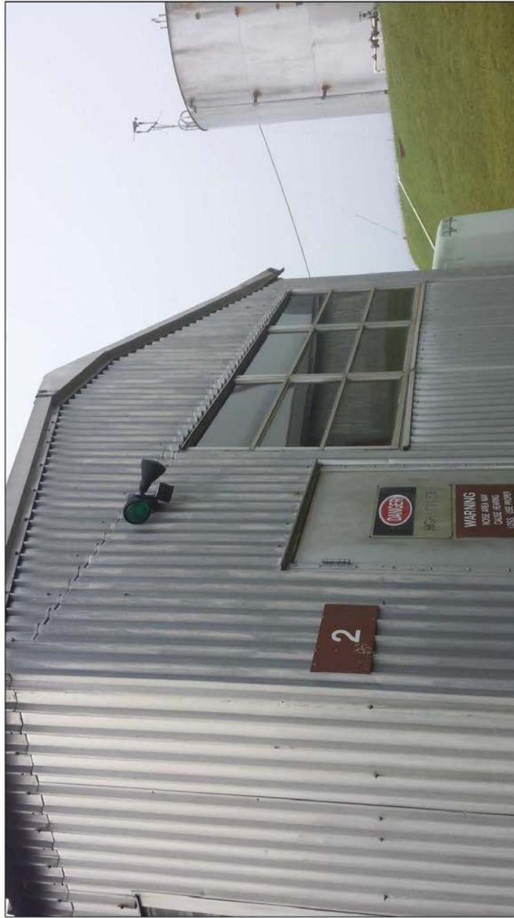
Building 2_Flood Light 2: Two green bulbs, both with shielding and motion detection, facing north (close up).
