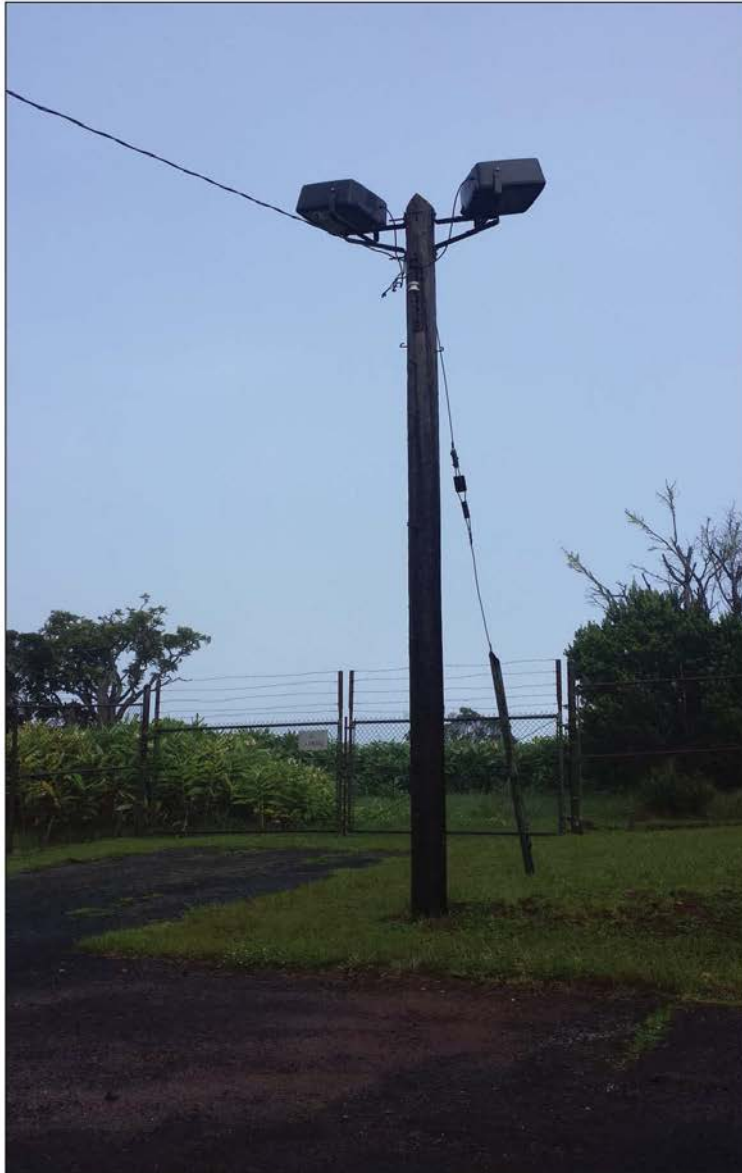
Perimeter Light_K: Two green bulbs, with full shielding, located in the most western corner of the installation.
