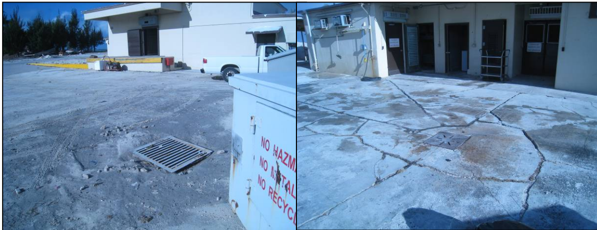
These photographs show the inlets east of Building 1104 (Dining Hall) that drain to Outfall No. 7.
