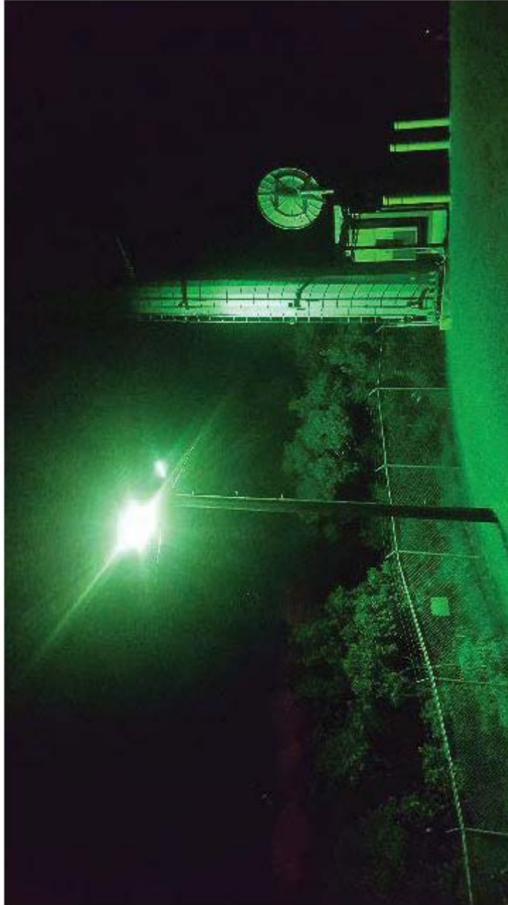
Perimeter Light_C: One green bulb, with full shielding (photo taken after the light was realigned in a downward position).
