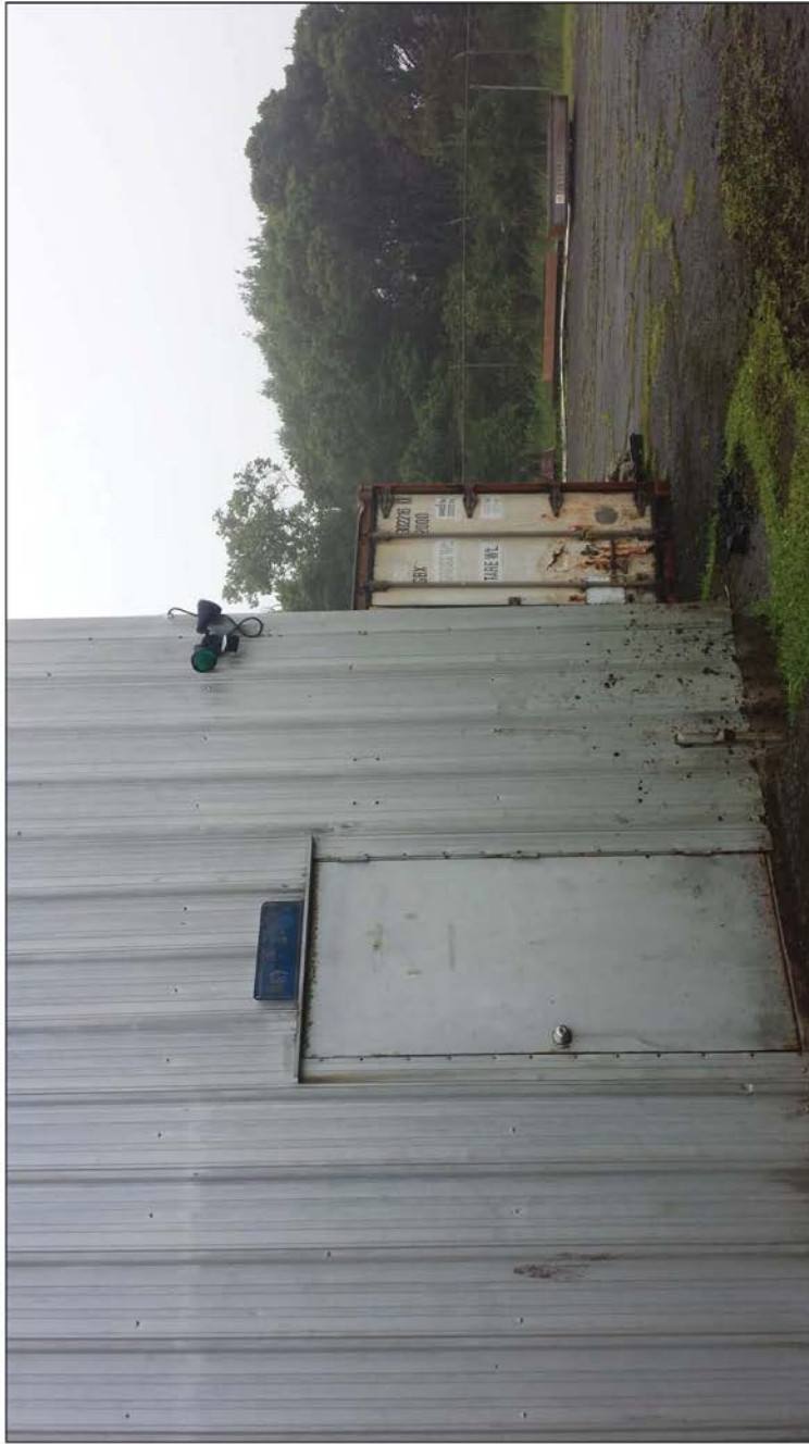
Building 5_Flood Light 2: Two green bulbs, both with shielding and motion detection.
