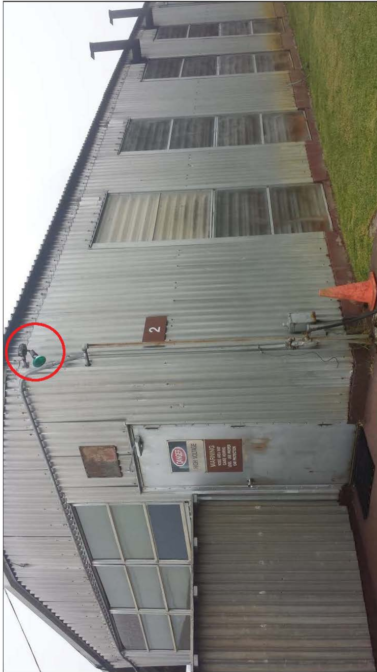
Building 2_Flood Light 1: One green bulb with no shielding or motion detection.
