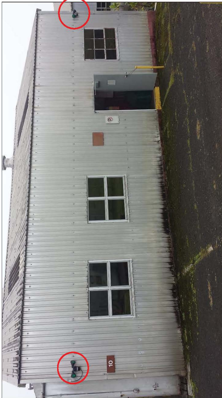
Building 10_Flood Lights 1 and 2: Two green bulbs each, both with shielding and motion detection.
