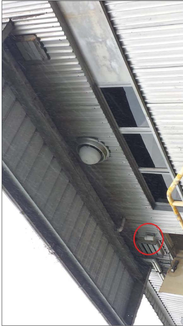
Building 1_Entryway Light 1: One white bulb, with no shielding and no motion detection (close-up), 2 nd floor.
