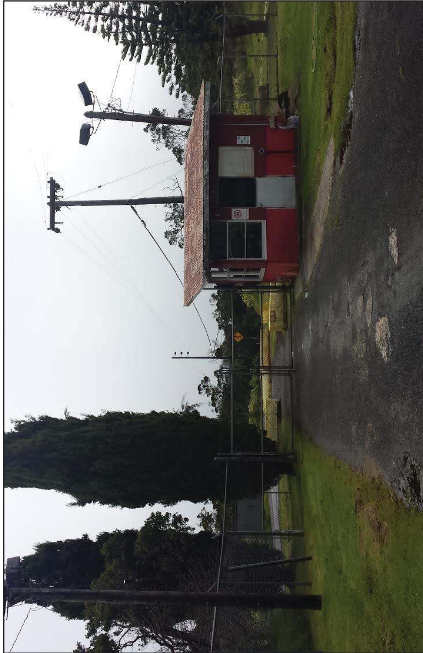
Perimeter Light_Q: Two green bulbs, with full shielding, located immediately southwest of the guard shack.
