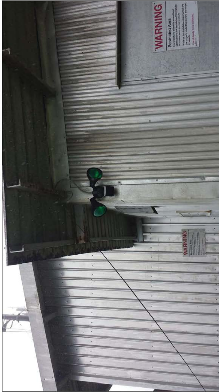
Building 1_Flood Light 1: Two green bulbs with motion detection (close up).
