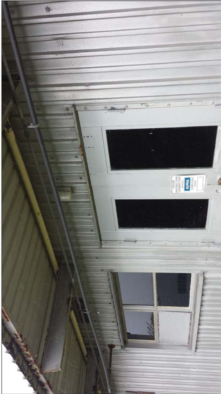
Building 1_Entryway Light 2: One white bulb, no shielding and no motion detection (close-up), 1 st floor, southeast – facing.
