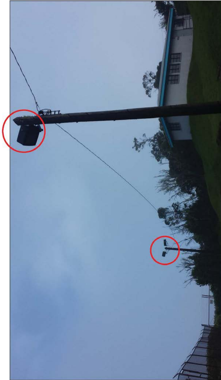
Perimeter Light_K: Two green bulbs, with full shielding (circle on the left).
