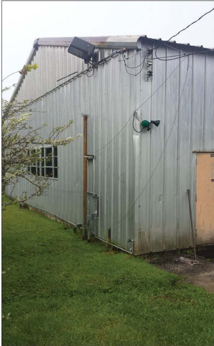
Building 5_Flood Light 3: Two green bulbs, both with shielding and motion detection.
