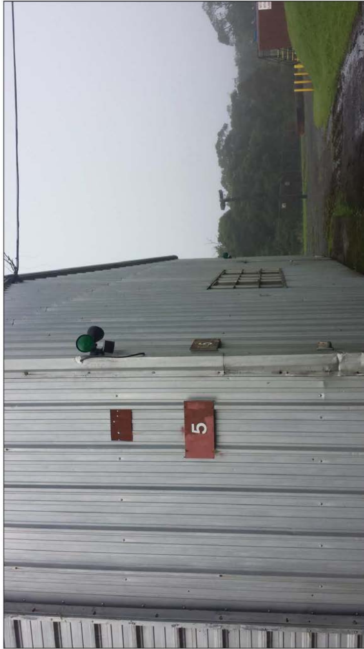
Building 5_Flood Light 1: Two green bulbs both with shielding and motion detection.
