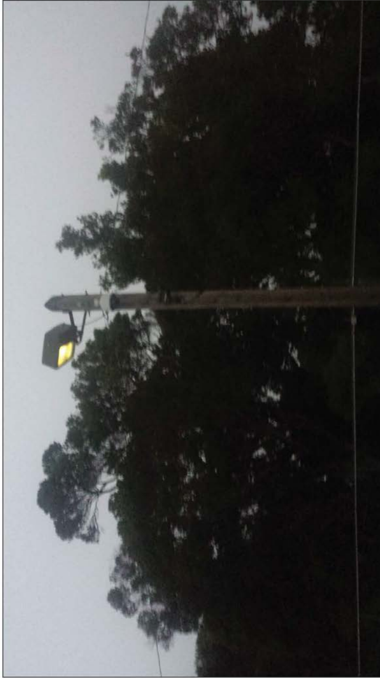
Perimeter Light_B: One green bulb, with full shielding and green light illuminated.
