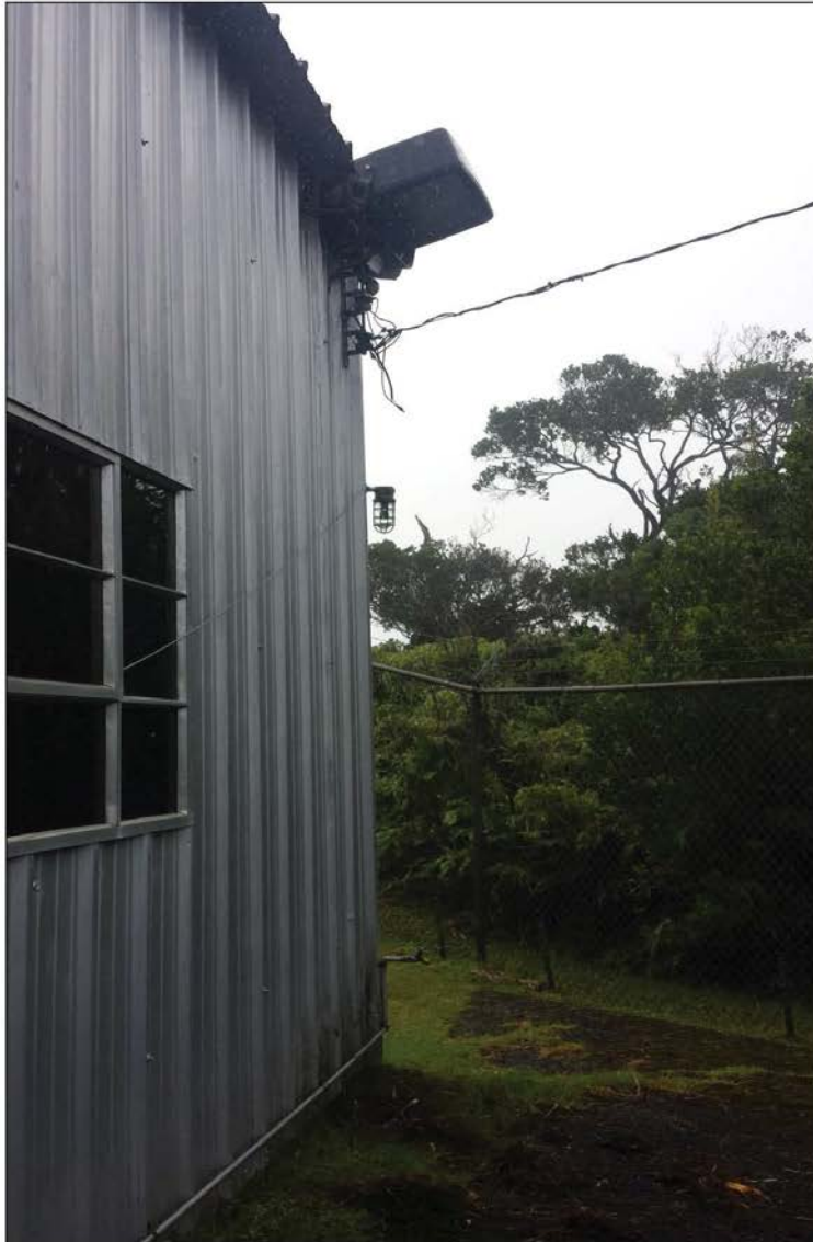
Perimeter Light_O: One green bulb, with full shielding, mounted on the southwest corner of building 5.
