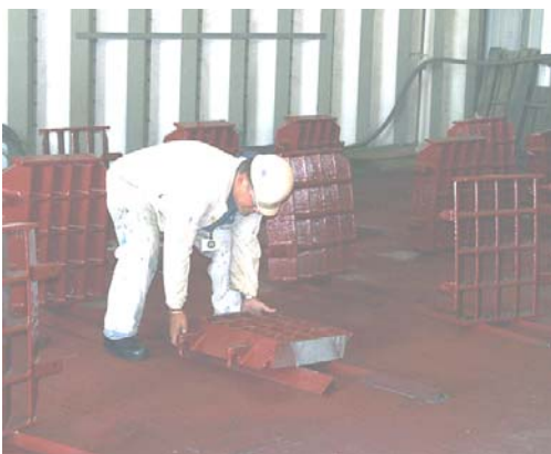
Figure 3: Employee flipping grate
