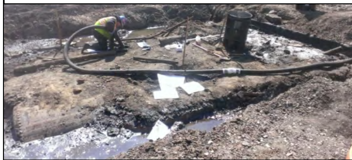
Figure 8: A worker pumps out tanks prior to removal. These tanks were "discovered" during construction
