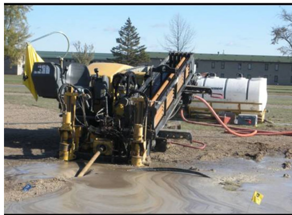
Ground source heat pumps: The pumps were installed for the new Education Center addition currently being constructed at Camp Ripley. This technology has decreased energy consumption by 45% at other facilities.
