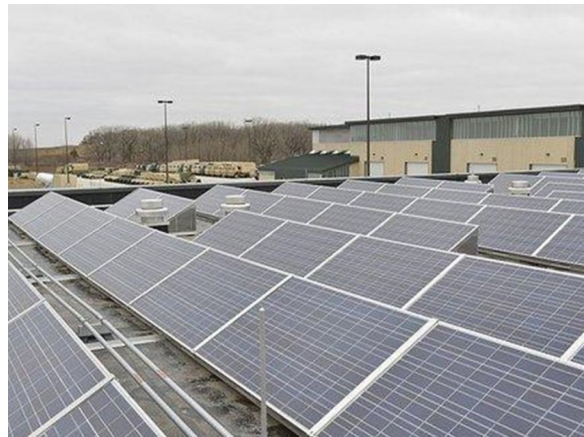
Solar PV and Solar Thermal equipment at AHATS: This solar PV system was designed to provide 6.5% of the facilities electrical requirements.
