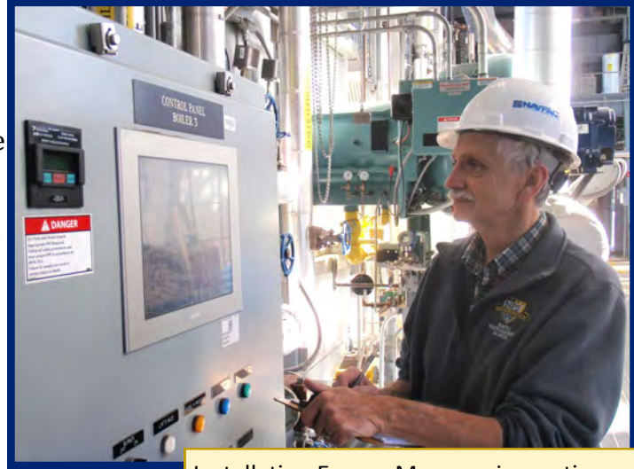
Installation Energy Manager inspecting high-efficiency boiler monitoring system.
