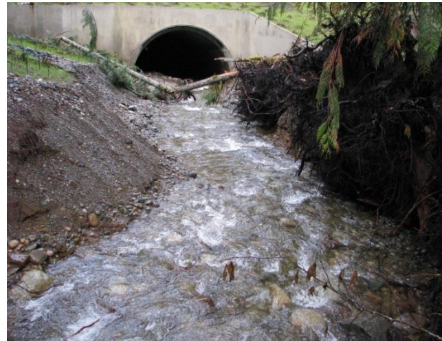
NAVBASE Kitsap replaced a 48" diameter culvert with a $6M 20' wide natural bottom tunnel to provide passage for ESA-listed salmon species.
