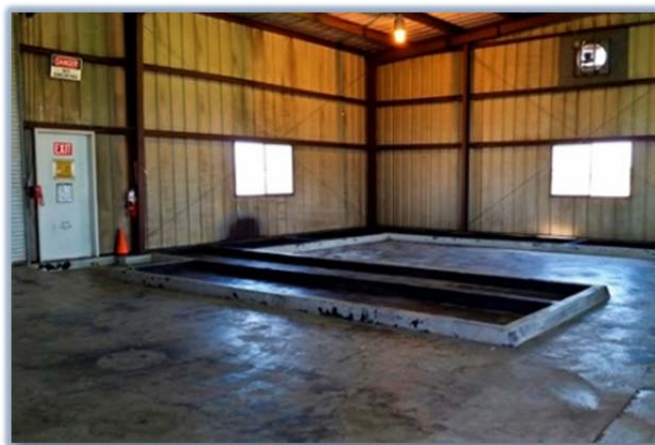
Bldg. 605 Hazardous Waste Storage after hazardous waste was removed and the building cleaned and power-washed.
