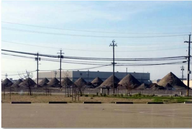
Crushed concrete from demolition of warehouse flooring to be used as soil erosion control.
