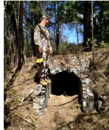
A Marine documents current conditions of a tunnel that was used to connect two World War II era aircraft revetments at Marine Corps Training Area Bellows.
