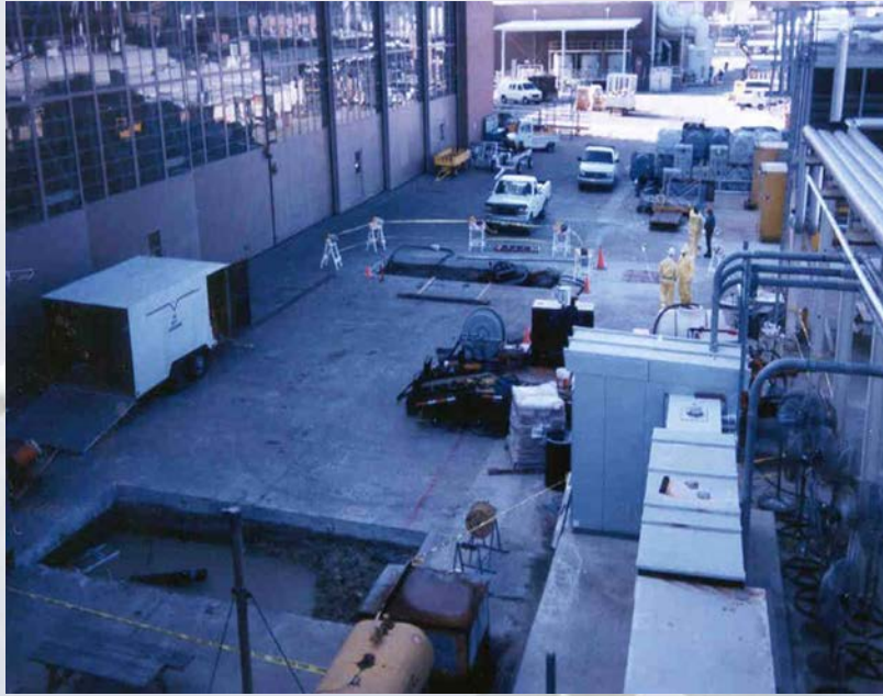
Restoration activities in Cherry Point's highly congested industrial area require careful coordination to limit impacts on production and avoid damage to utilities and infrastructure.
