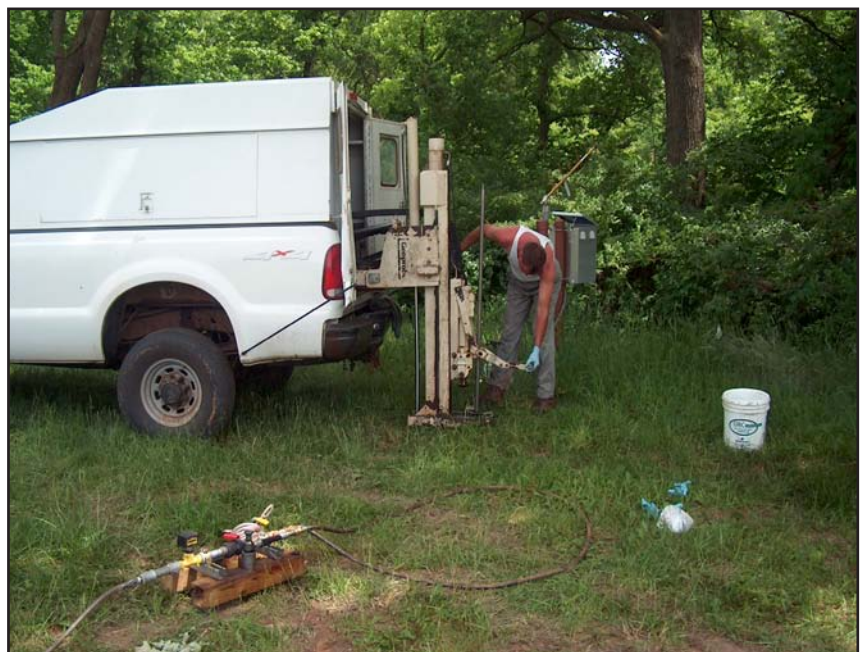
A geoprobe and small pump were used during the CAP-18 soybean oil injection.
