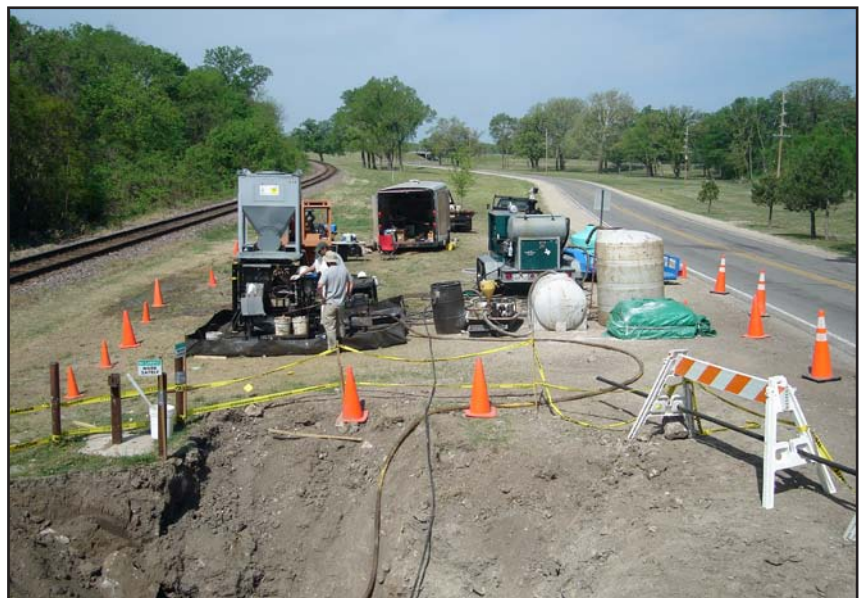
The IRP team used high-pressure permanganate injection equipment to treat the groundwater of the Dry Cleaning Facilities Area.
