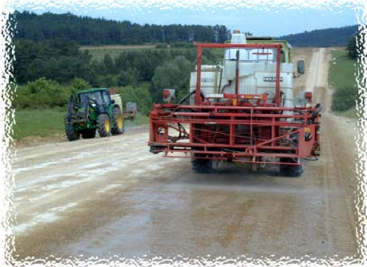
Calcium chloride was applied to roads by a local contractor to reduce the amount of environmental dust caused by tanks.
