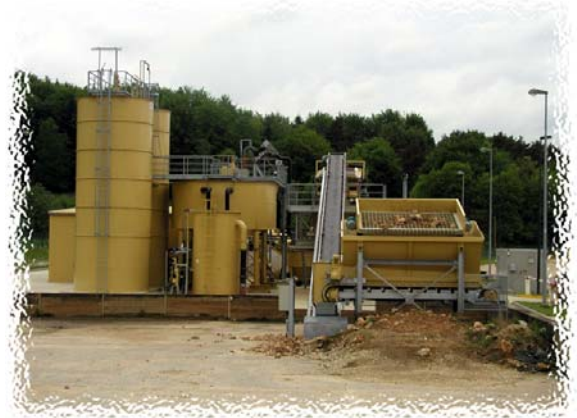
The innovative new sludge treatment facility will reduce the amount of sludge for disposal by approximately 80%.
