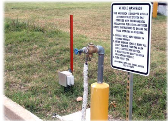
TXARNG deployed a prototype design using a diverter valve that is operated hydraulically and is activated by the water pressure.
