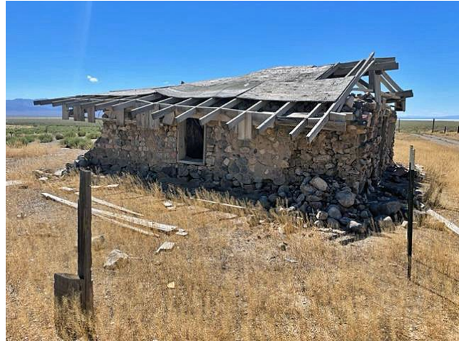
Boyer Ranch House Constructed in the 1860s, Oldest Building in Churchill County, and Located on Navy Fee Lands
