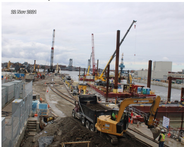
In FY 2022 and 2023, the ER Program provided technical and regulatory support on two major projects within ER boundaries at PNSY: Consolidation and Construction of the Paint, Blast, and Rubber Facility (P293) and Modernization and Expansion of Dry Dock 1 (P381), pictured above.
