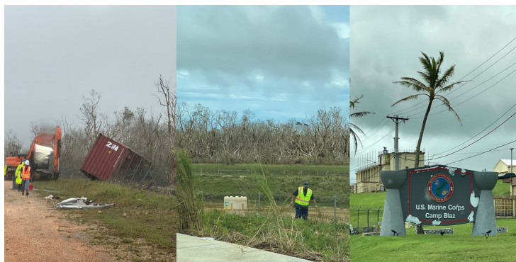
This mosaic depicts the challenges of post-Typhoon Mawar recovery, with heavy damage to infrastructure, debris from nearby forests and construction areas, and damaged water and power infrastructure. Center: Richard Salas (Physical Scientist).
