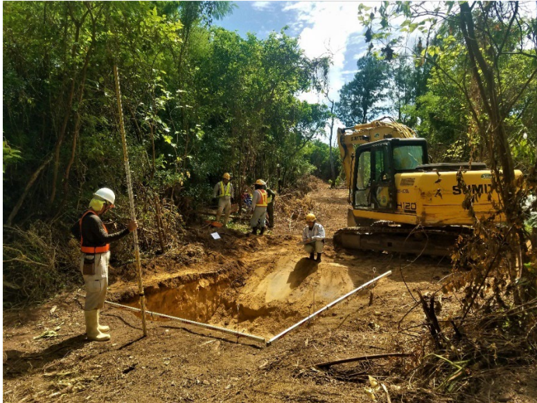
Example of contractors excavating large scale pits during the testing at Kin Blue Beach.
