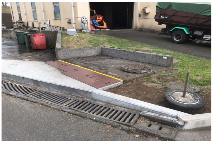
Yokota AB constructed a concrete curb to ensure wash water flowed to the oil water separator before entering the stormwater drainage system.
