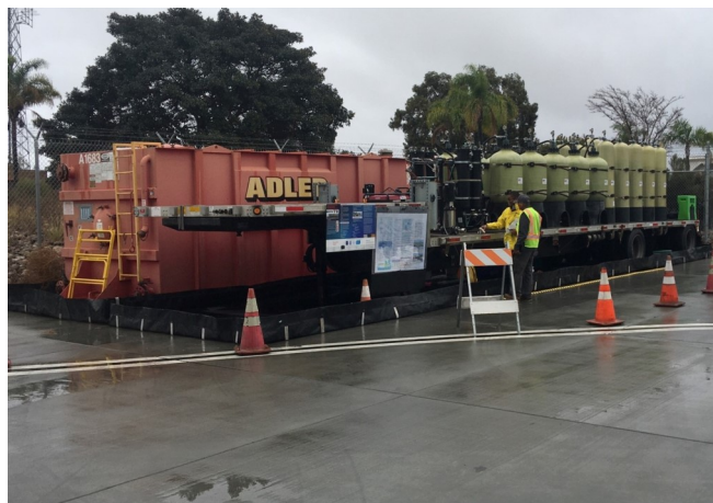
MCAS Miramar EMD staff employ their mobile trailer-mounted treatment system to remove PFAS contaminants from AFFF-impacted wastewater. Water is processed through the system vessels of organoclay, granular activated carbon, ion-exchange resin media, and colloidal scavenger resin. After sampling, staff discharge the wastewater to the sanitary sewer.
