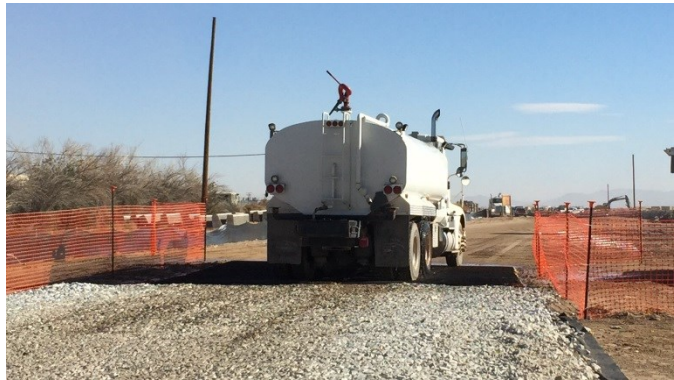
To mitigate dust, personnel use watering trucks to spread water over base roadways. A project is now in place to use recycled asphalt that generates less dust so less water is required therefore increasing resiliency.
