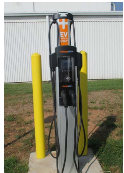
Figure 3 – Electric Vehicle Charging Station
