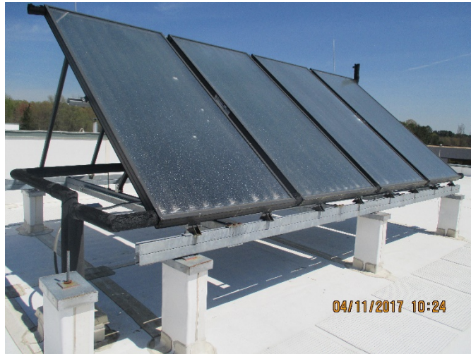
Figure 2 - Solar Water Preheat Panels at Dahlgren
