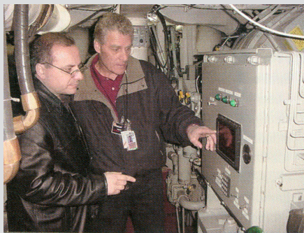
Mr. Joe DiDominic (left) and Mr. Dan DiVigense of NSWCCD-SSES Code 9153 look at the new microprocessor-control panel on AC plant #2 aboard the USS Laboon (DDG-58).
